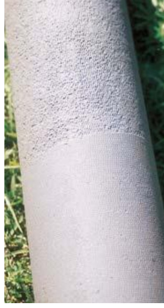
This grit blasted ductile iron pipe was buried for over 11 years in aggressive soil. The left hand side of pipe was polyethylene sleeved, the right hand side left bare.
