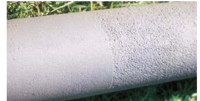
This grit blasted ductile iron pipe was buried for over 11 years in aggressive soil. The left hand side of pipe was polyethylene sleeved, the right hand side left bare.
